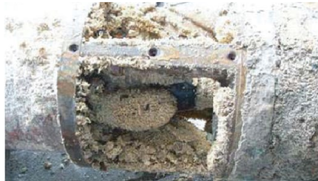
Sea life growth inside the pump intake and on the pump shaft
